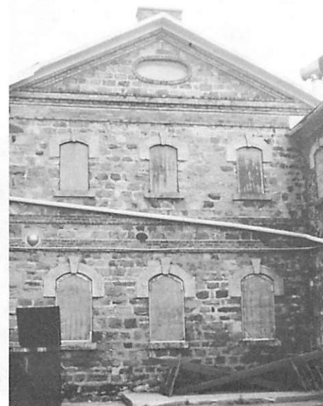
East wall of jail showing stonework and brick band courses and pediment outline.
